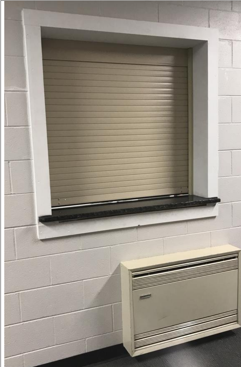
CONCESSIONS WINDOW IS NOT ACCESSIBLE – SILL IS AT 42”
