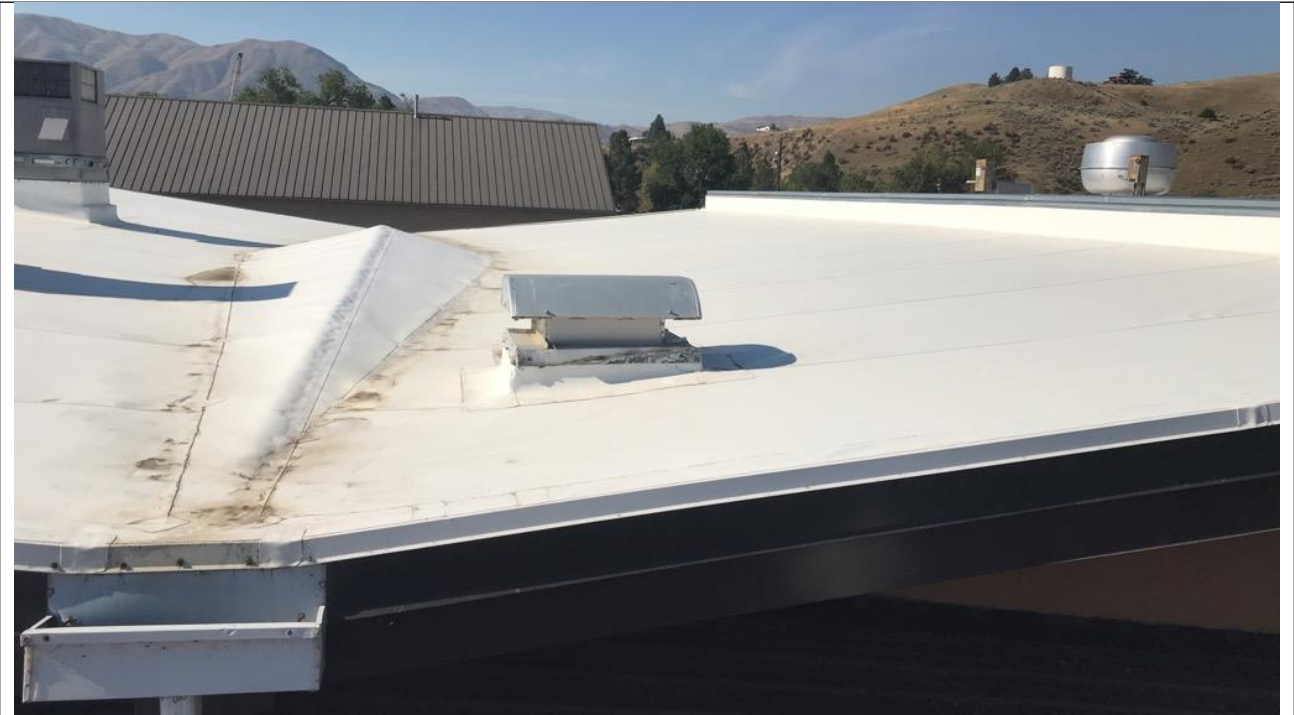
SINGLE PLY MEMBRANE ROOF AT CAFETERIA IS IN GOOD CONDITION. DRAIN TO LOWER ROOF NEED REPAIR TO PREVENT LEAKING
