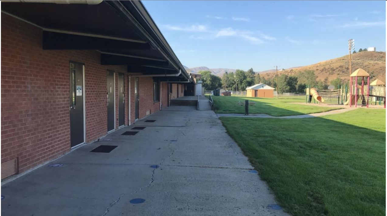
WALKWAY AT ELEMENTARY / RAMP AND HANDRAIL DOES NOT MEET ADA REQUIREMENTS.
