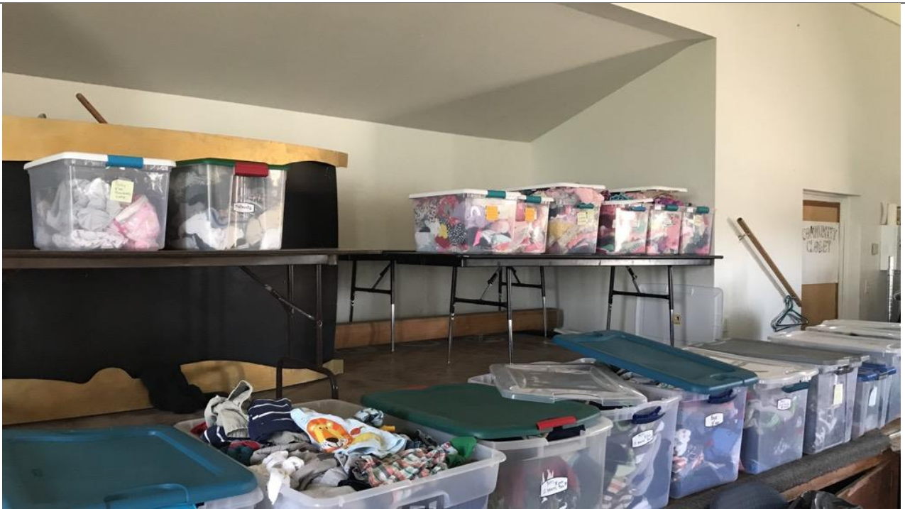
STAGE / RAISED PLATFORM – NO ADA ACCESS
