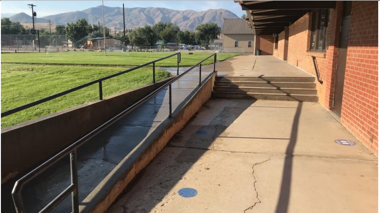
RAMP AND HANDRAILS DO NOT MEET ADA. CONCRETE IS SPALLING / CRACKING
