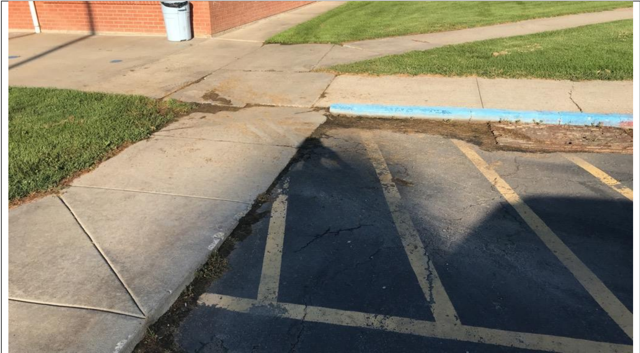
ADA SIDEWALK ACCESS ISSUES AT MAIN PARKING LOT BY ELEMENTARY
