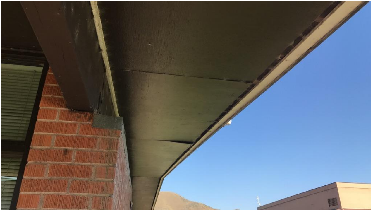
WOOD SOFFIT MATERIAL DAMAGED AND SHOWING AGE FROM WATER DAMAGE
