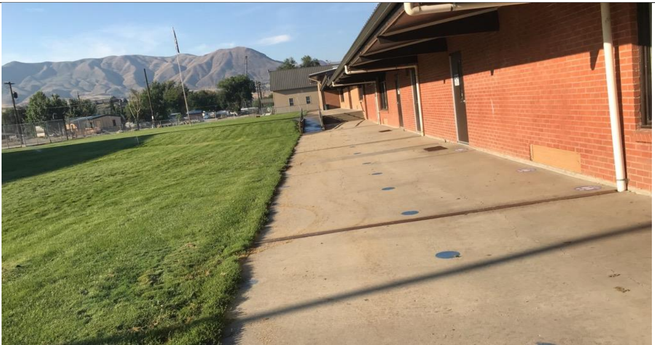
WALKWAY AT EAST SIDE OF ELEMENTARY / DOWNSPOUT DRAINAGE ISSUES UNDER CONCRETE SLAB AND CONNECTION POINT TO DOWNSPOUT
