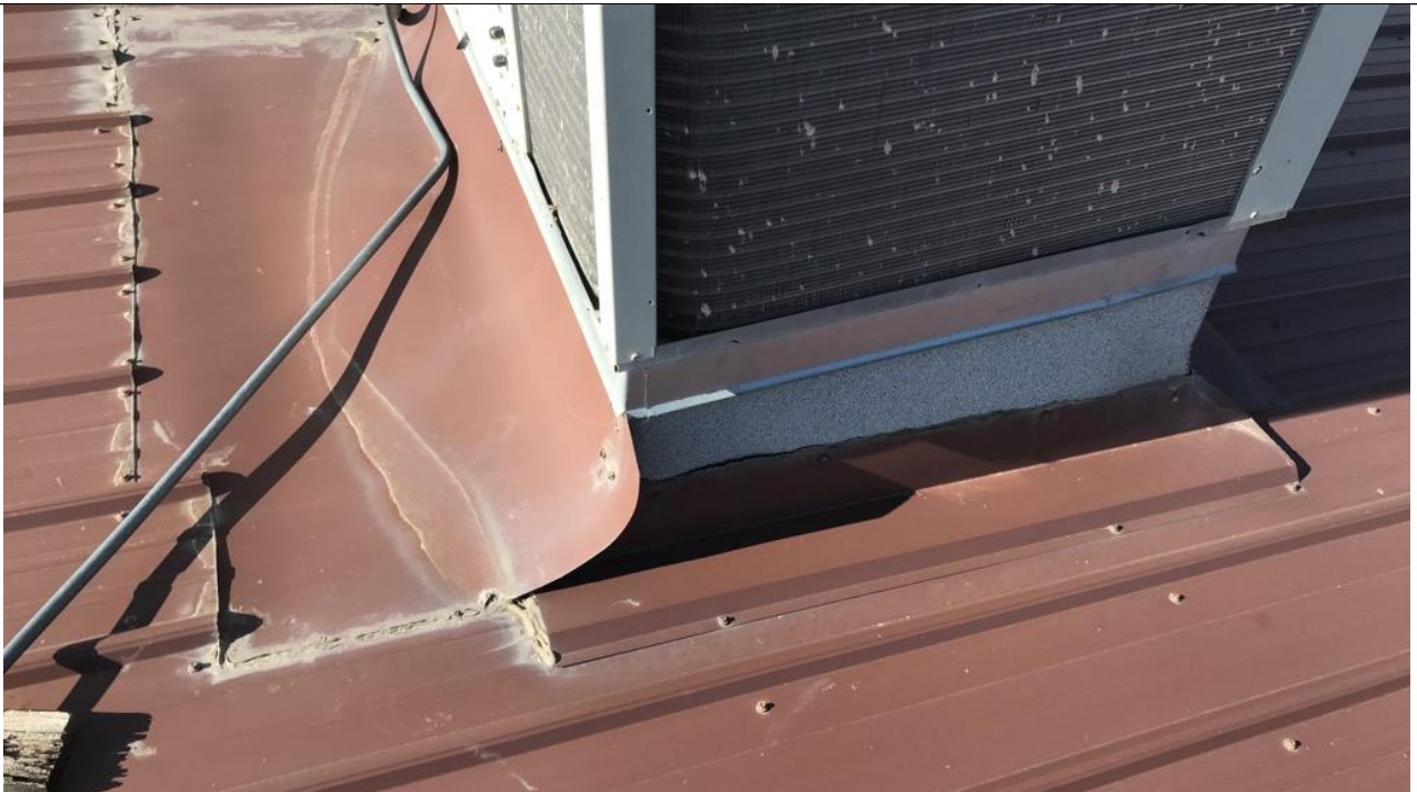
PENETRATIONS AT HVAC UNITS ARE IN POOR CONDITION
