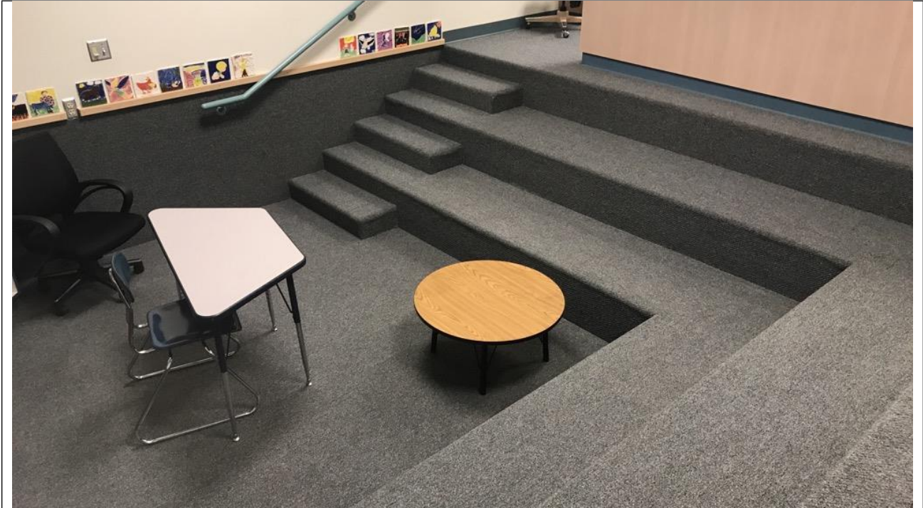
RECESSED READING AREA DOES NOT MEET ADA REQUIREMENTS
