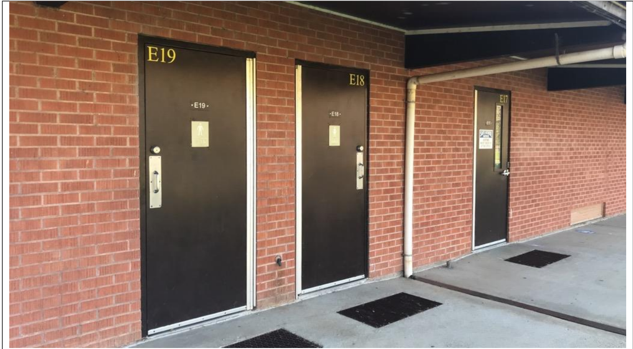
EXTERIOR DOWNSPOUTS TO SOLID FLOOR DRAIN CAUSING DRAINAGE ISSUES
