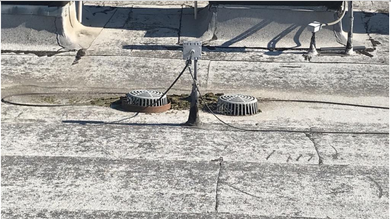
ROOF DRAIN AND OVERFLOW / SURROUNDED BY HEAT TAPE
