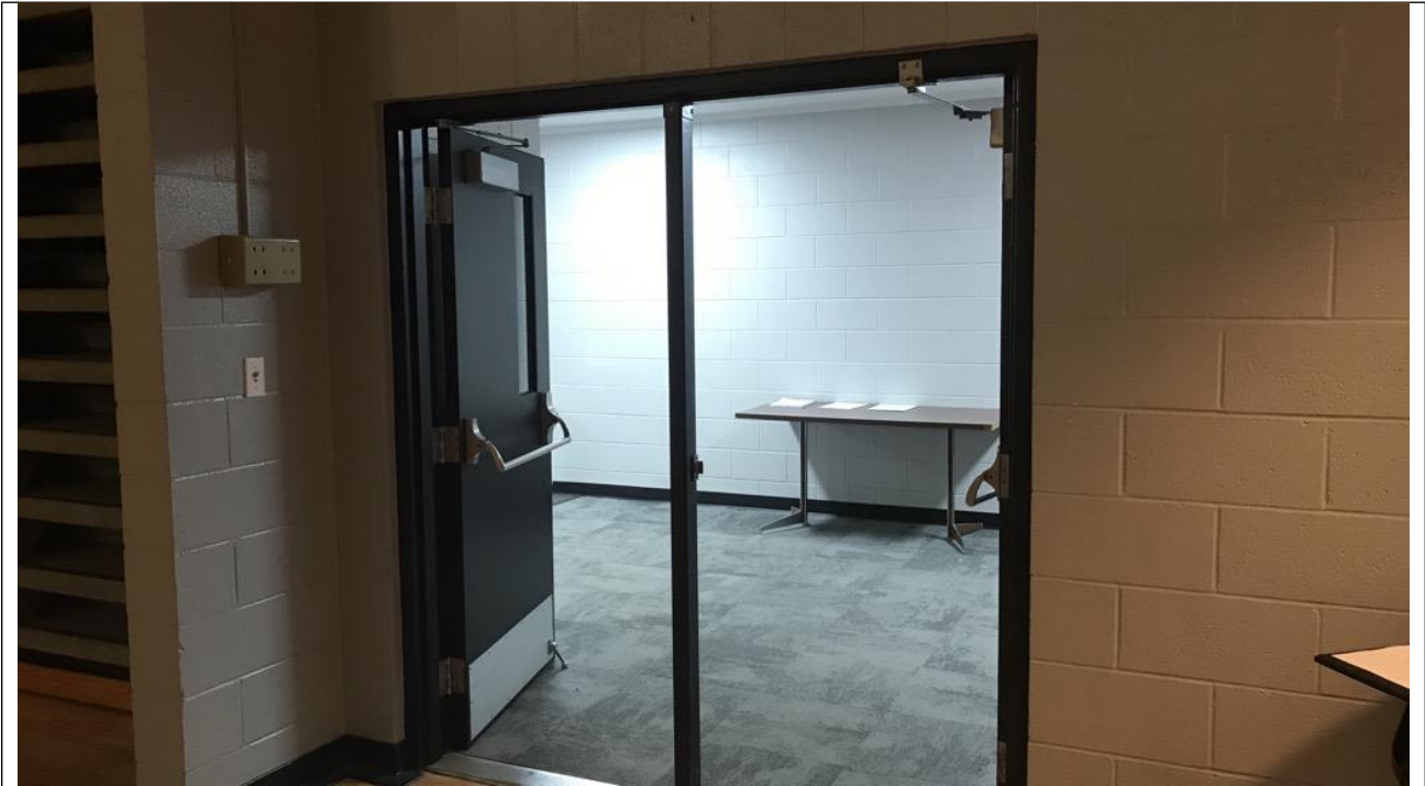
EXIT DOORS / HARDWARE MEETS ADA REQUIREMENTS / COULD BE UPGRADED
