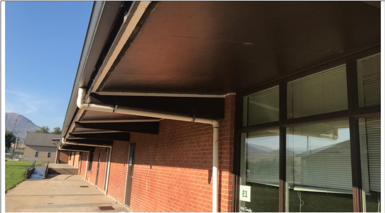
OVERHANG WITH DOWNSPOUTS. WATER DAMAGE AT SOFFIT FROM DRAINAGE
