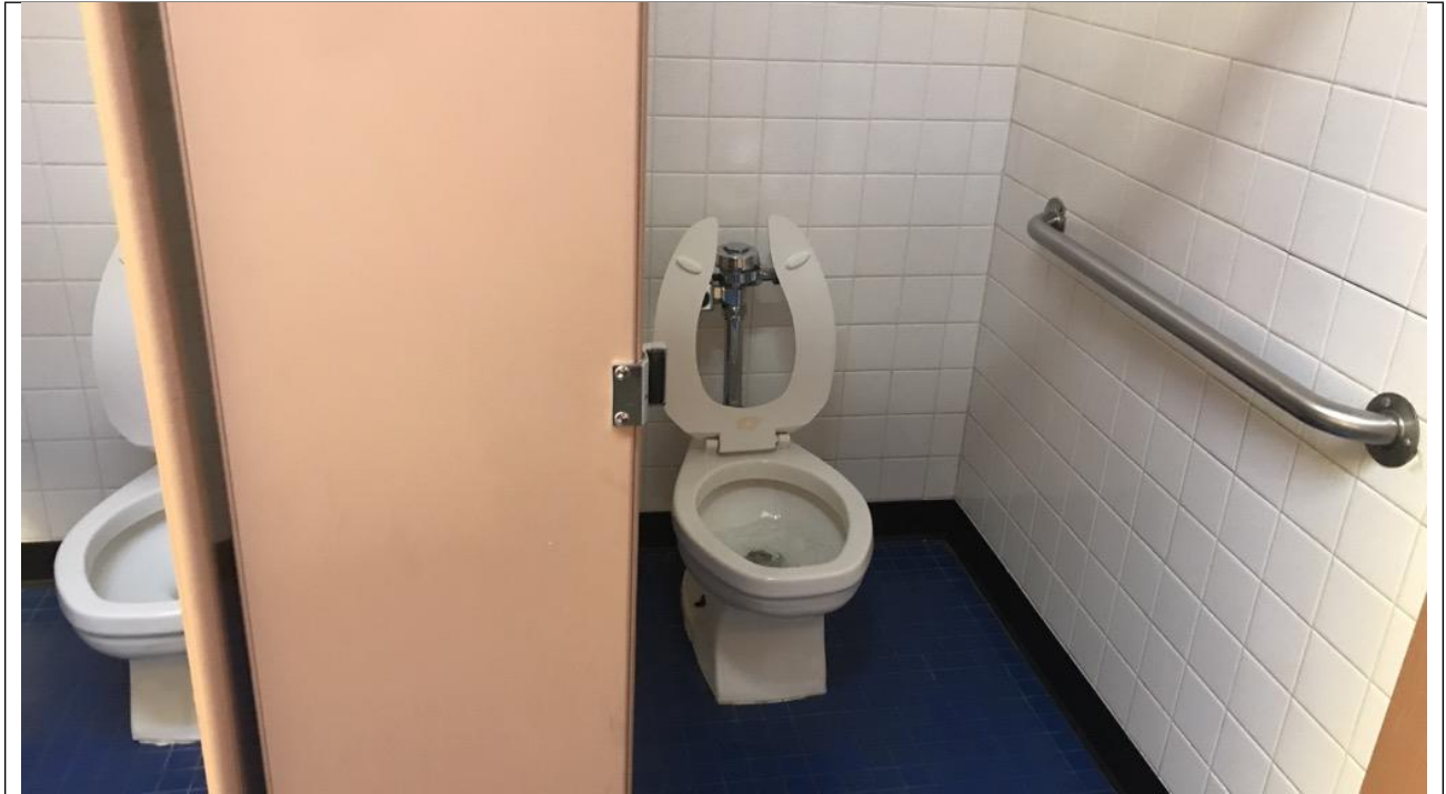
RESTROOMS / NO ACCESSIBLE STALL
