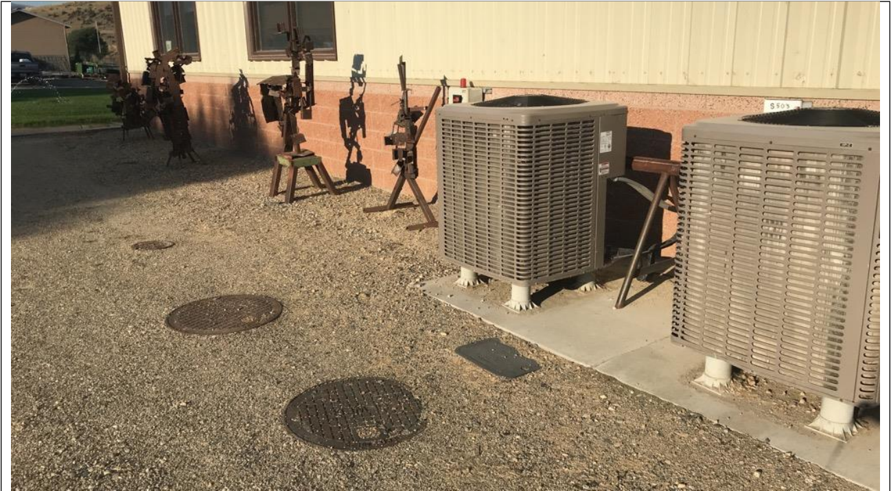
MECHANICAL UNITS AT CTE / UNDERGROUND UTILITIES / SEWER-WATER
