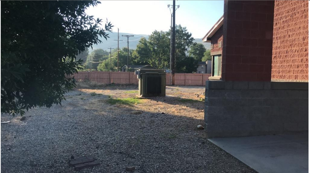
POWER TRANSFORMER AT MIDDLE SCHOOL
