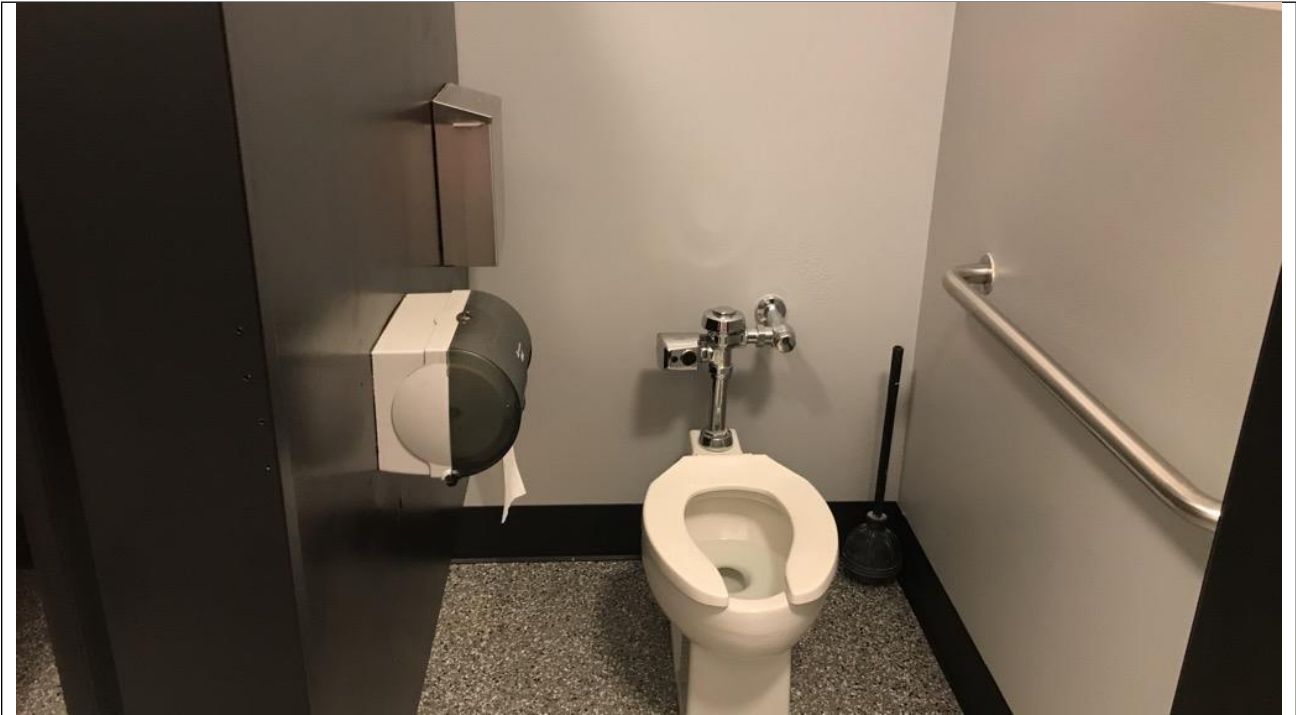
STALLS DO NOT MEET ADA REQUIREMENTS
