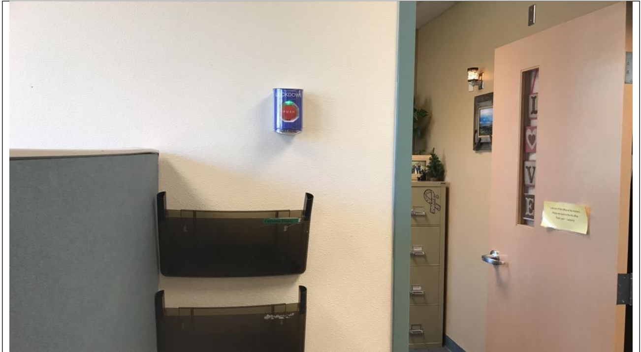
EMERGENCY LOCK DOWN BUTTON
