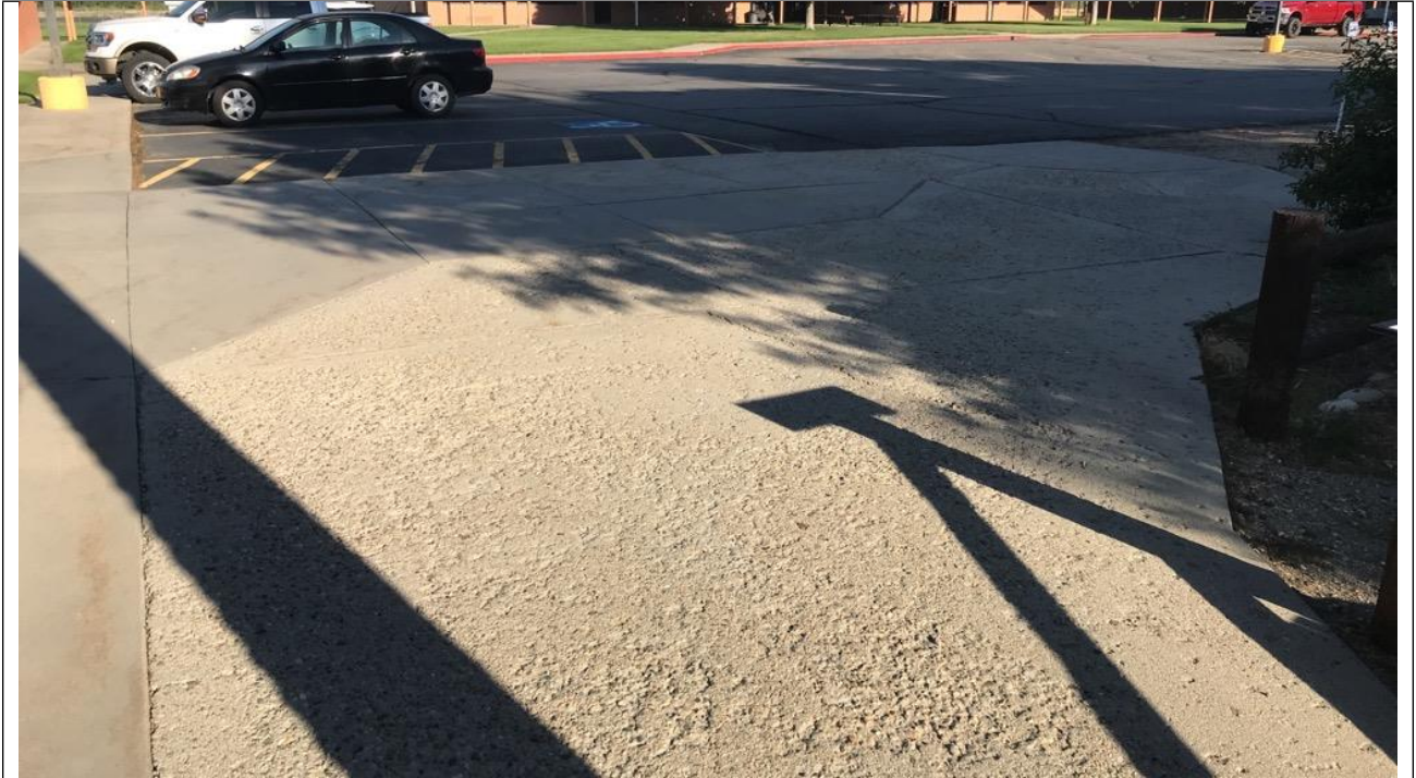
SIDEWALK LEADING TO MAIN ENTRY / CONCRETE IS SPALLING
