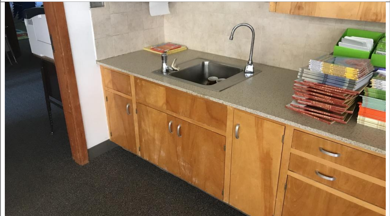
SINK CABINETS DO NOT MEET ADA REQUIREMENTS
