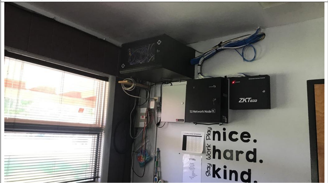
IT RACKS AT RESOURCE CLASSROOM
