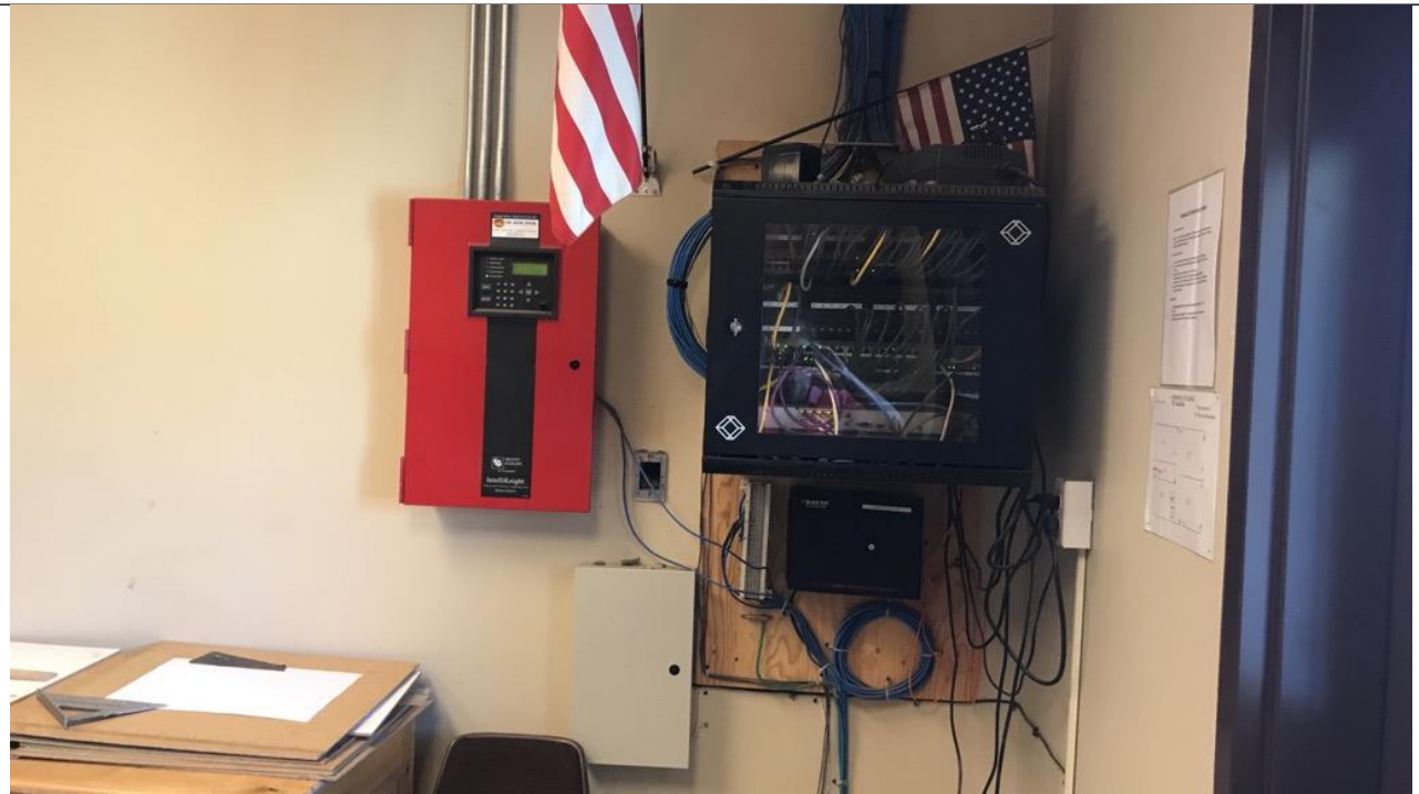
FIRE ALARM AND DATA RACK
