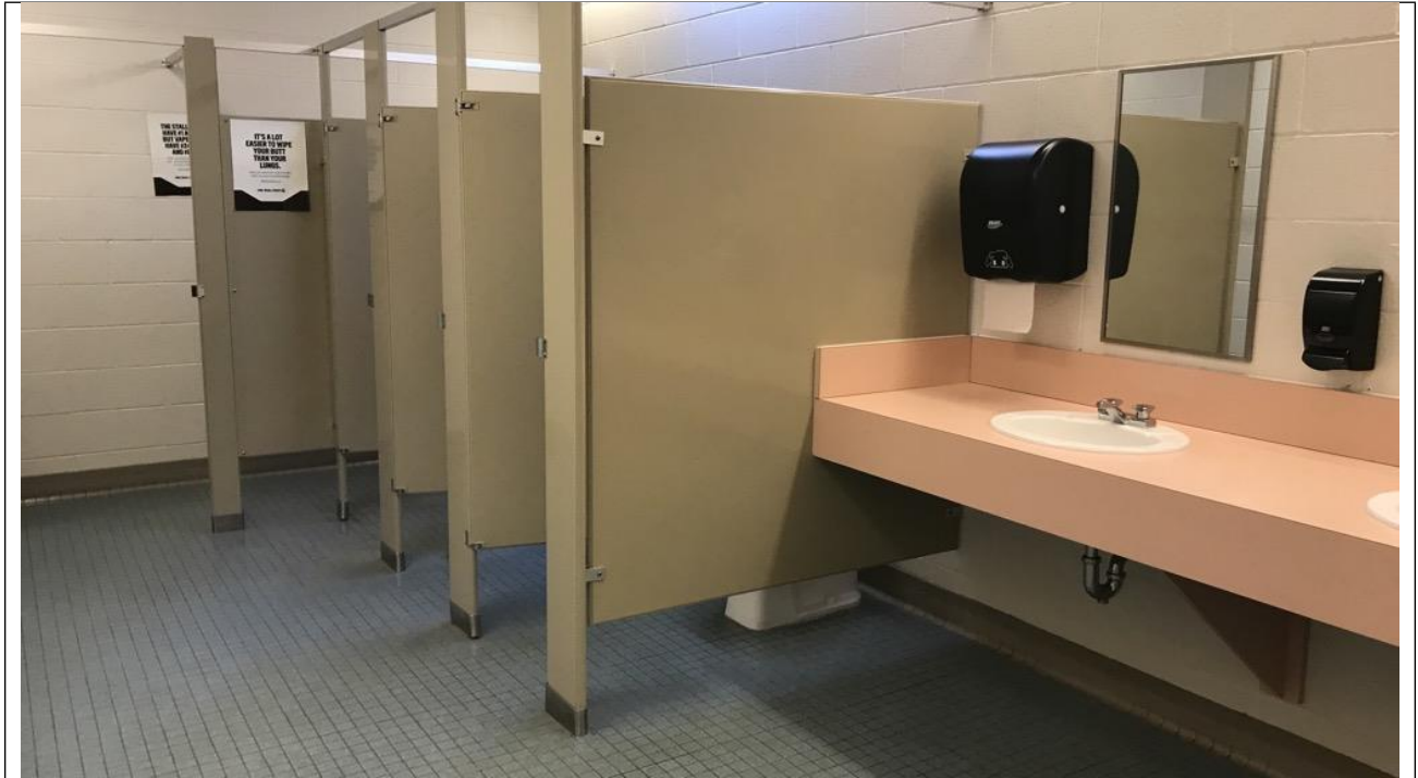
PUBLIC RESTROOMS / SINKS DO NOT MEET ADA HEIGHT REQUIREMENTS
