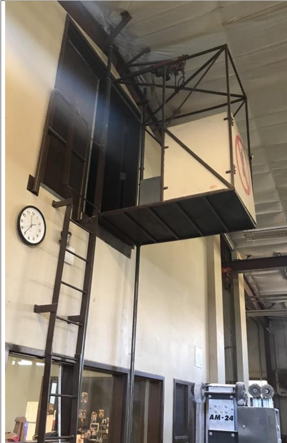
DUMBWAITER / LIFT IS NOT OPERATIONAL LADDER ACCESS TO MECHANICAL PLATFORM
