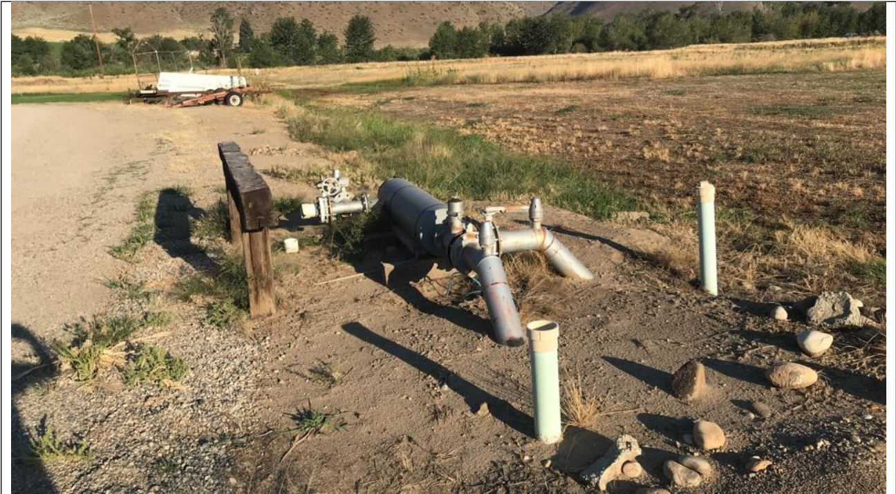
IRRIGATION SYSTEM AT NORTH ACCESS ROAD
