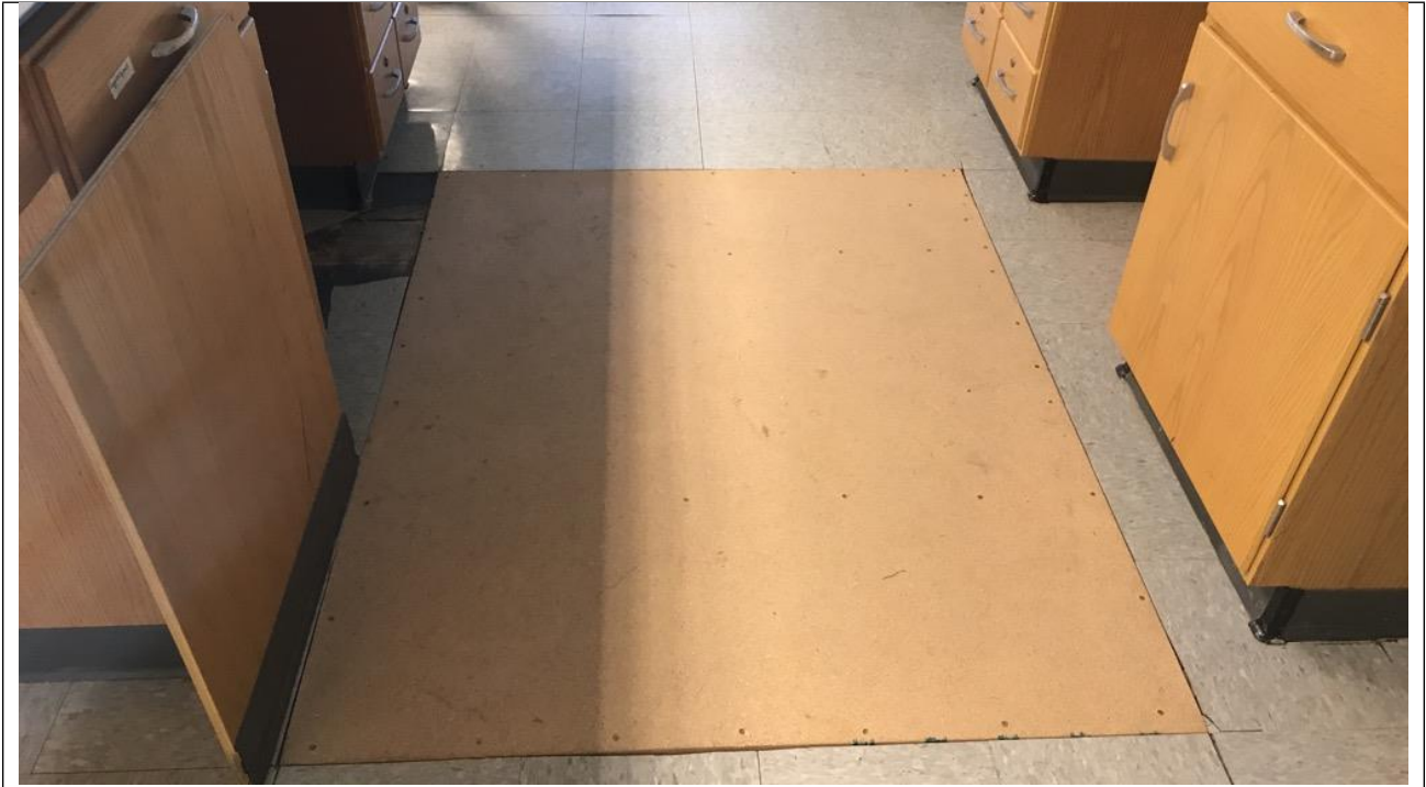
WATER DAMAGE FROM WATER LEAK / CHEMISTRY CLASSROOM
