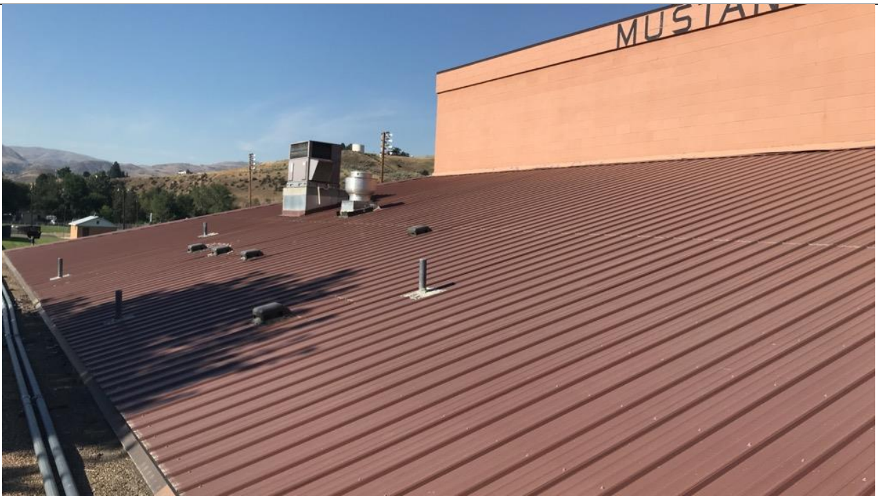
ROOF TOP MOUNTED HVAC EQUIPMENT
