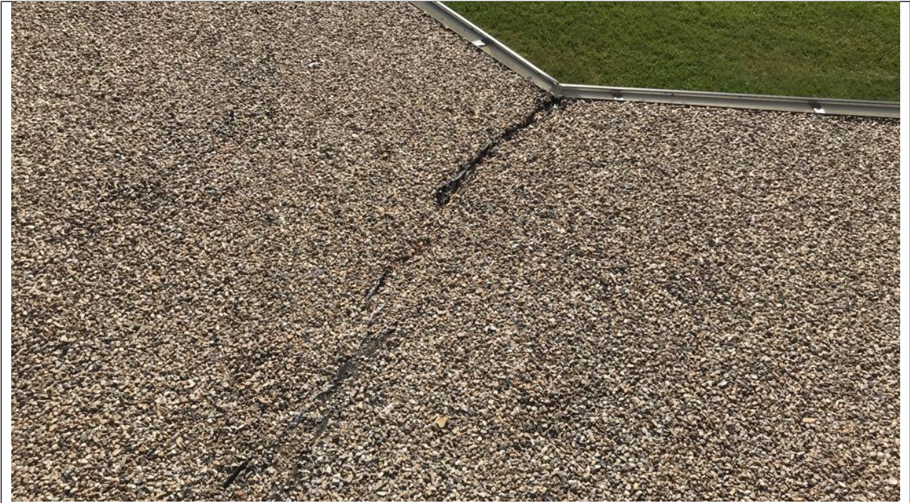
GRAVEL COVERED BUILT UP ROOFING – FLAT / SHOWING WEAR IN MANY LOCATIONS
